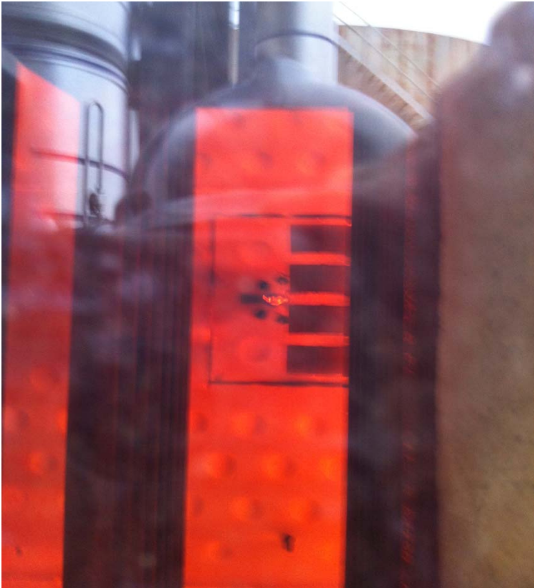
Figure 6. Flameless Firing. View from across heater.
